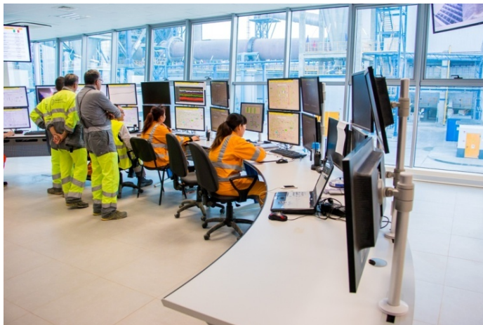
Central Control Room of CBMI Bulgaria Project
